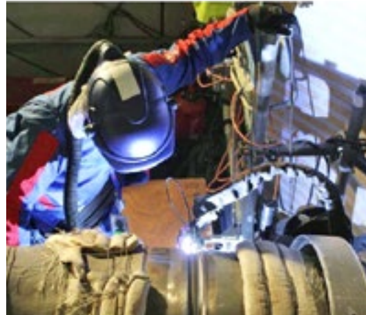
Implementation of the orbital TIG process – weld on the main secondary system
